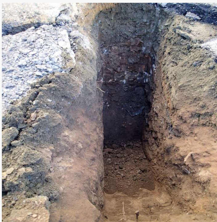
Photo 30: Soil profile at test pit location TP14. ACM cement sheet fragment found in fill material at 0.5 mBGL.
